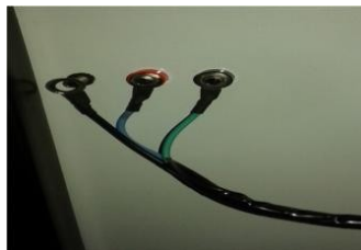
Figure 8. Assembly of Electrical Components and Wiring
